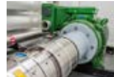
PUMPS AND MOTORS
